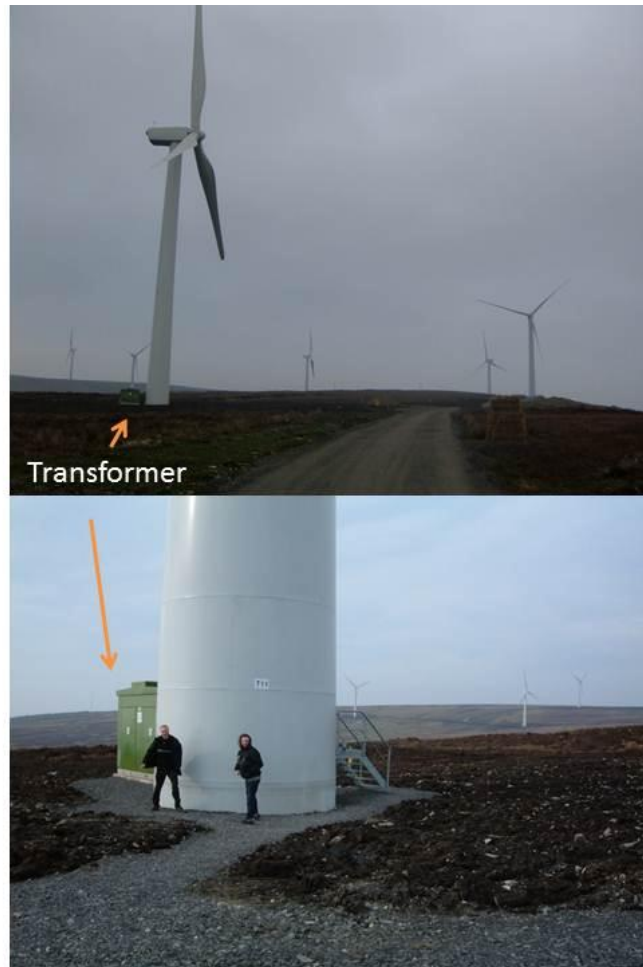
Plate 2-1: Photographs illustrating the turbine step-up transformer
