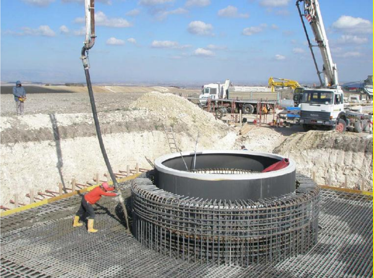
Plate 2-3: Concrete pouring of a turbine foundation – note the tower base collar in the foreground
