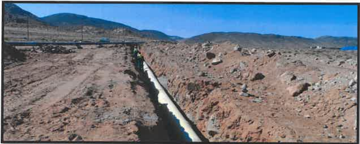
Photo 1: Typical below ground construction method (albeit for a much larger pipe), note construction footprint (in this case >30m)
