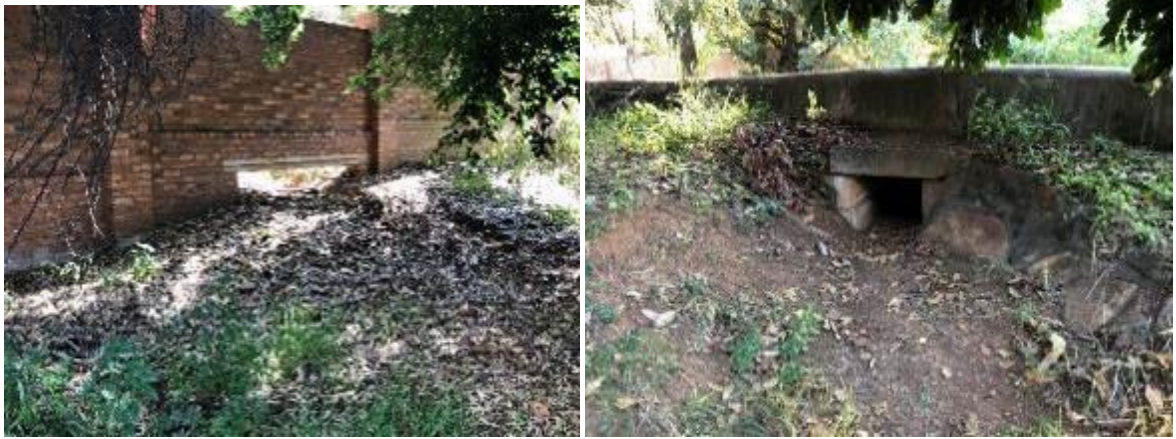
Figure 12: The opening in the boundary wall to Erf 348 and the culvert under the unnamed road.
