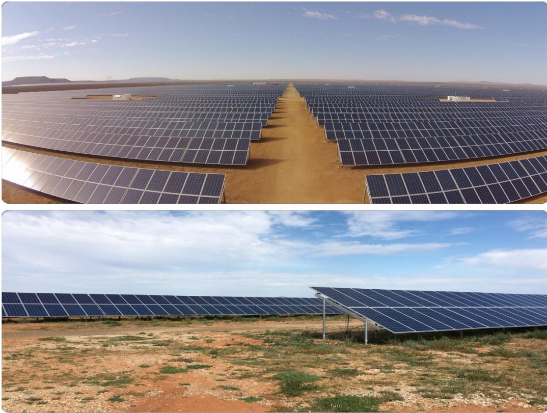
Figure 1: Photo showing an aerial view of PV panels & from ground level
