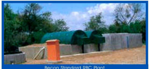
Becon Standard RBC Plant
