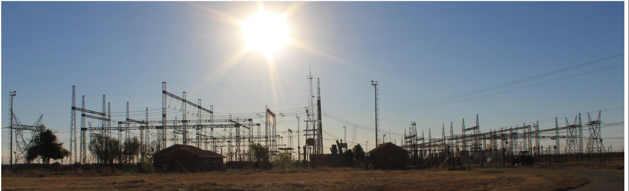
Theseus Main Transmission Station
