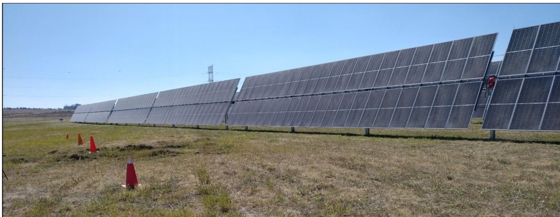
Figure 6. Front views of the PV arrays mounted on horizontal 1-axis tracker
