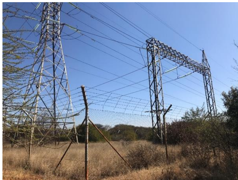
Figure 31: Substation identified on site
