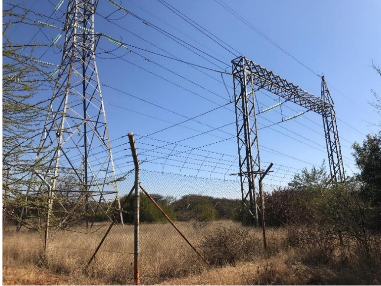
Figure 21: Substation identified on site
