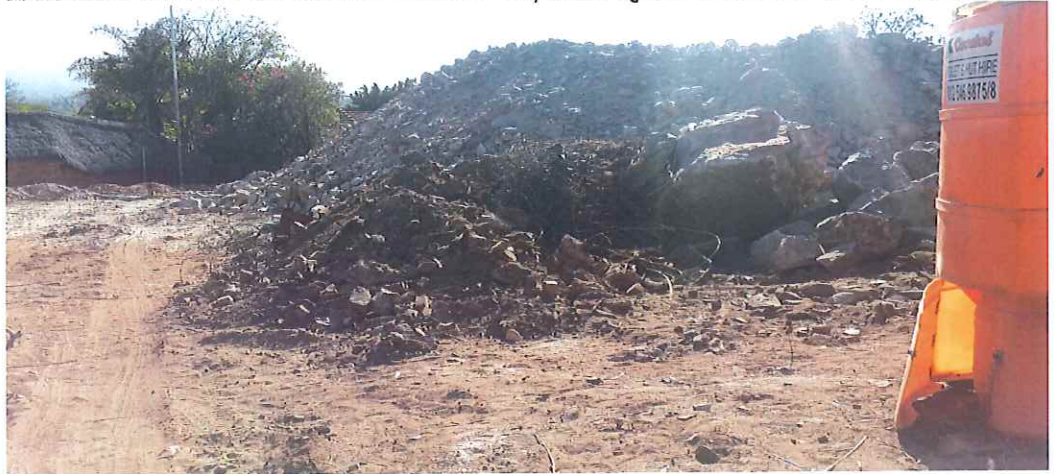
IMAGE 4: EXCAVATED MATERIAL AND WORKERS' ABLUTIONS ON SITE WITH EXISTING DWELLING HOUSE ON ERF 10/1011 QUEENSWOOD IN BACKGROUND
