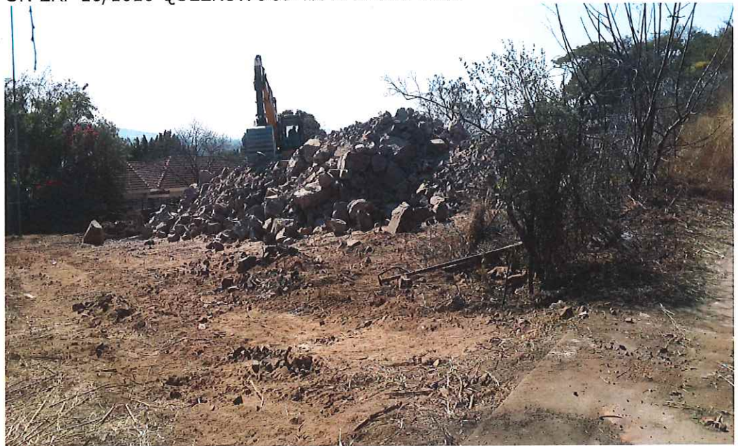
IMAGE 3: EXCAVATOR CLEARING THE SITE WITH EXISTING DWELLING HOUSE ON ERF 10/1010 QUEENSWOOD IN BACKGROUND
