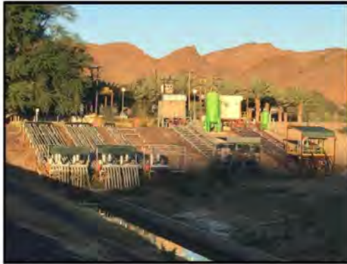
Figure 18. Pump station infrastructure with Vachellia erioloba on the left-hand side.
