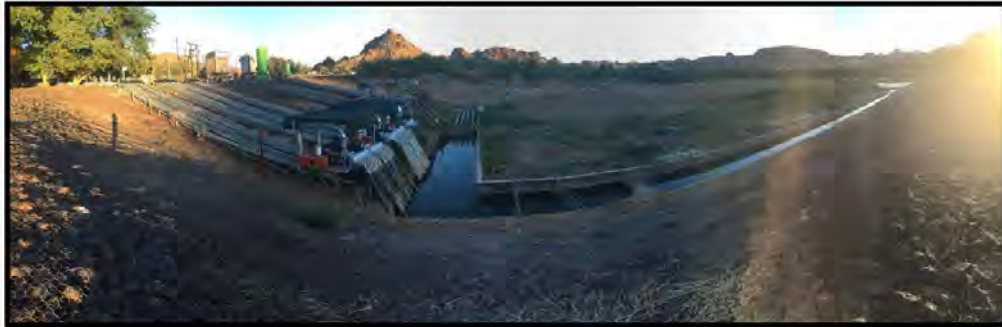
Figure 6: Intake and river pump station
