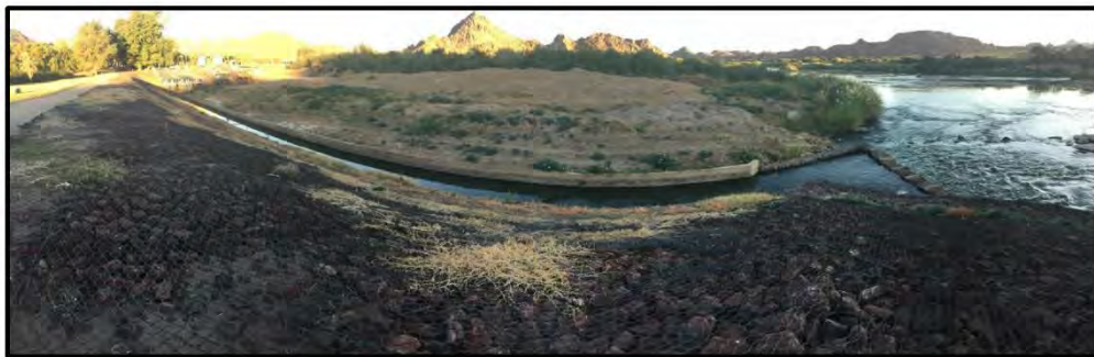
Figure 17. Overflow channel from the pump station within the alluvial zone of the Orange River.
