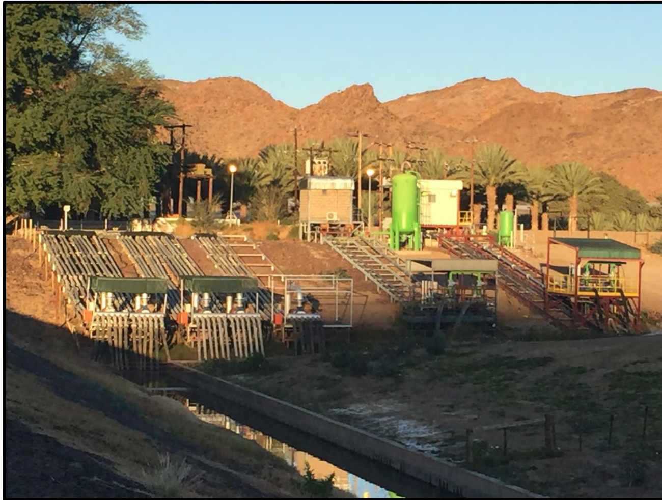
River pump station
