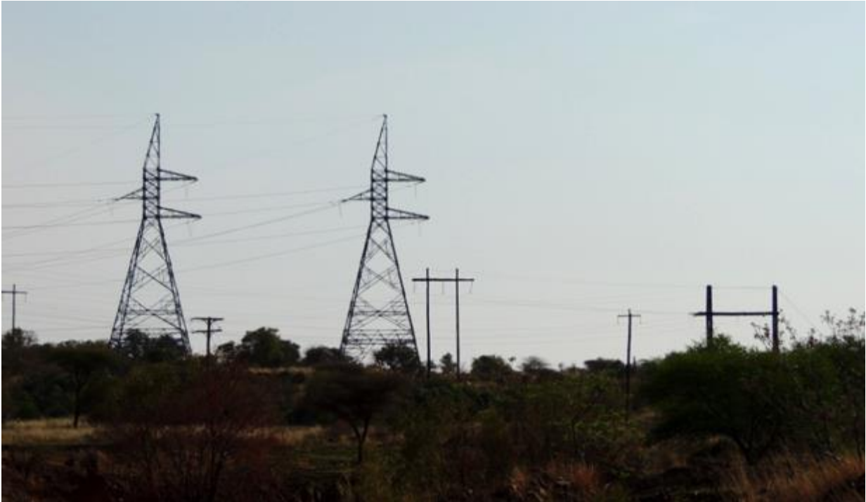
Figure 18: Photograph of the existing Eskom power lines routed to the south of the proposed corridor.
