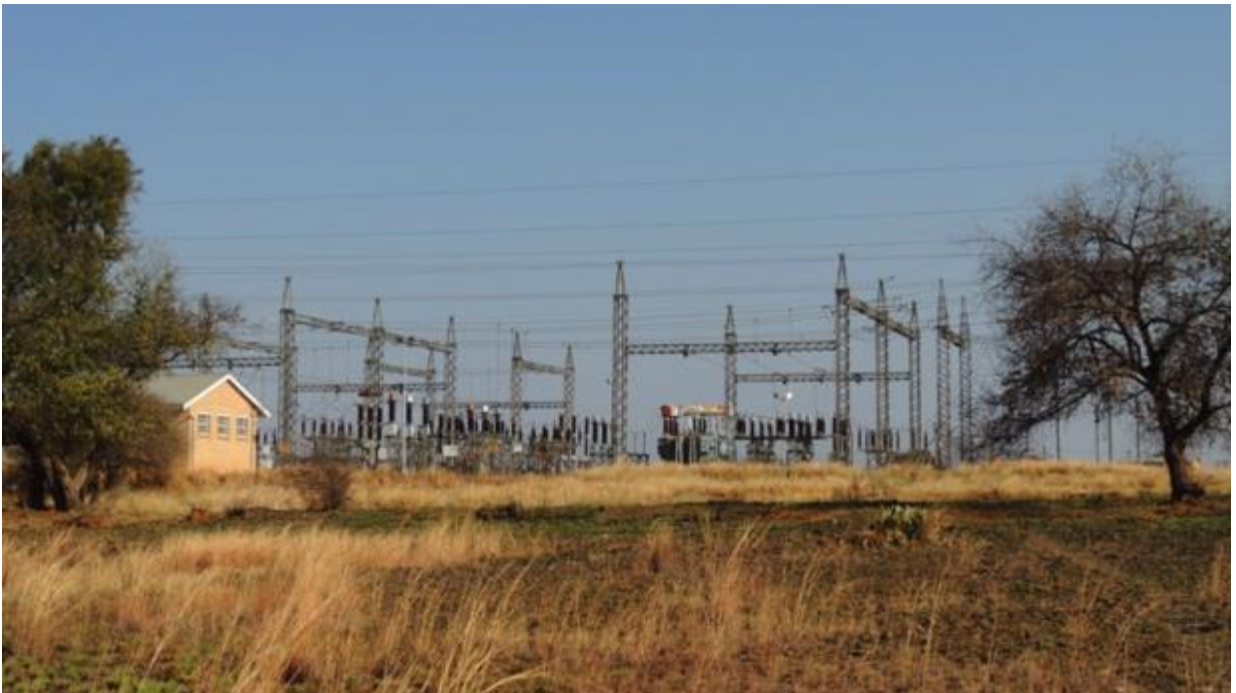
Figure 17: Photograph of the regional Eskom Substation
