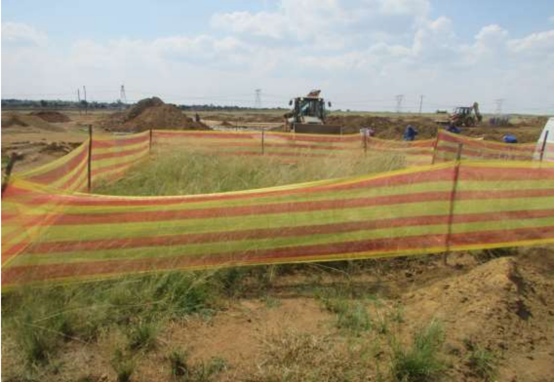
Figure 3: A view of the demarcated site with development activities around it visible.
