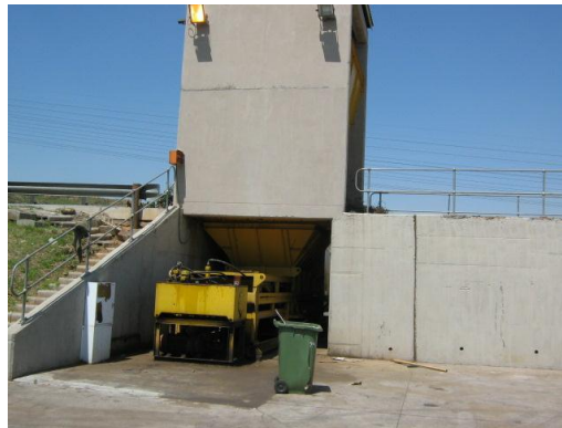
(b) Waste Compactor
