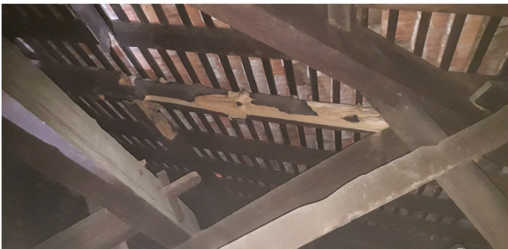
Damaged rafters in the library roof space
