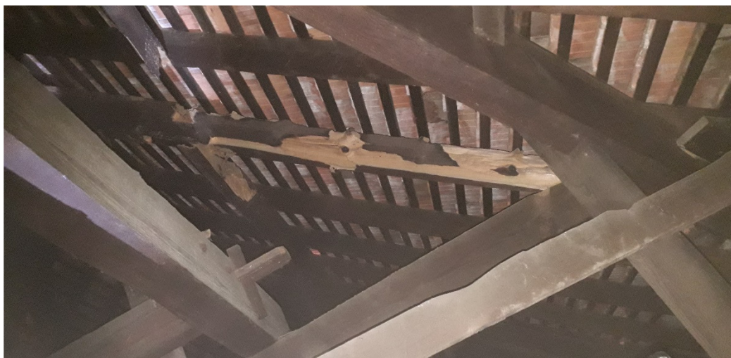
Damaged rafters in the library roof space
