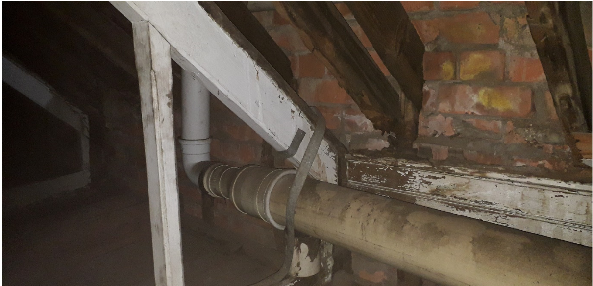
RW pipes in the roof above the library
