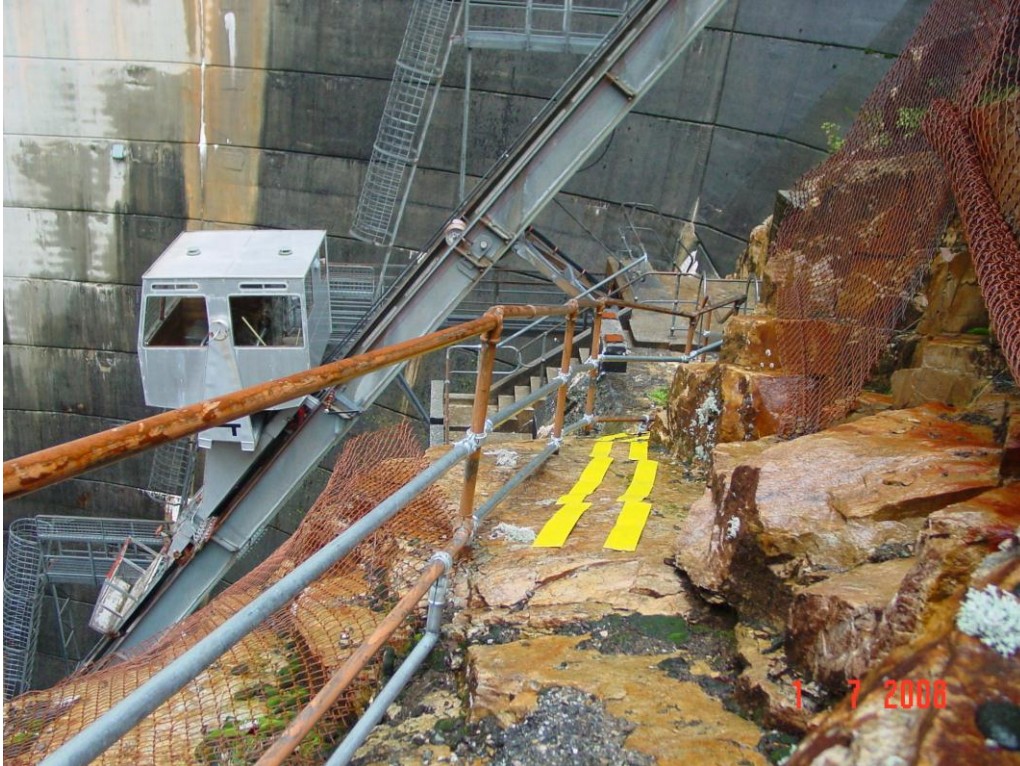
Figure 5: Example of a haulage-way utilised to remove spoil material from a dam construction site. (The skip in this photo is likely to be an open bin at the RVM site).
