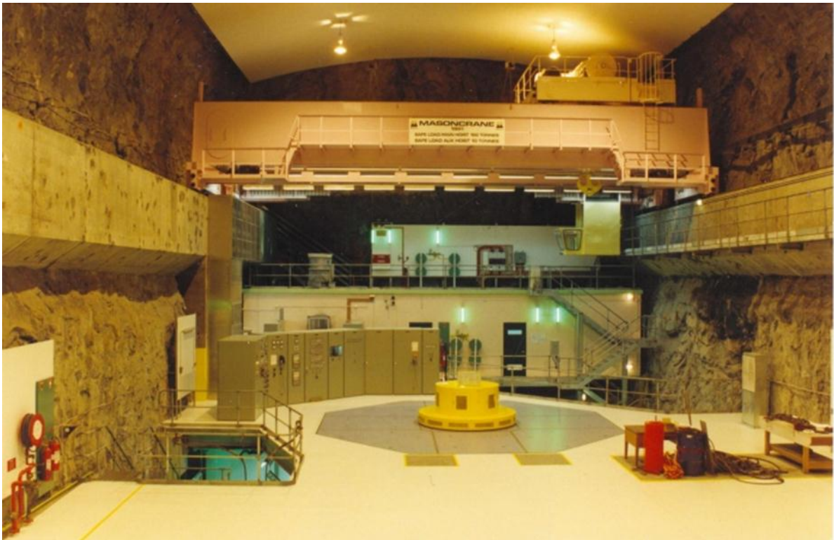
Figure 3: Underground power house. (Note for the proposed project the infrastructure would be smaller.)
