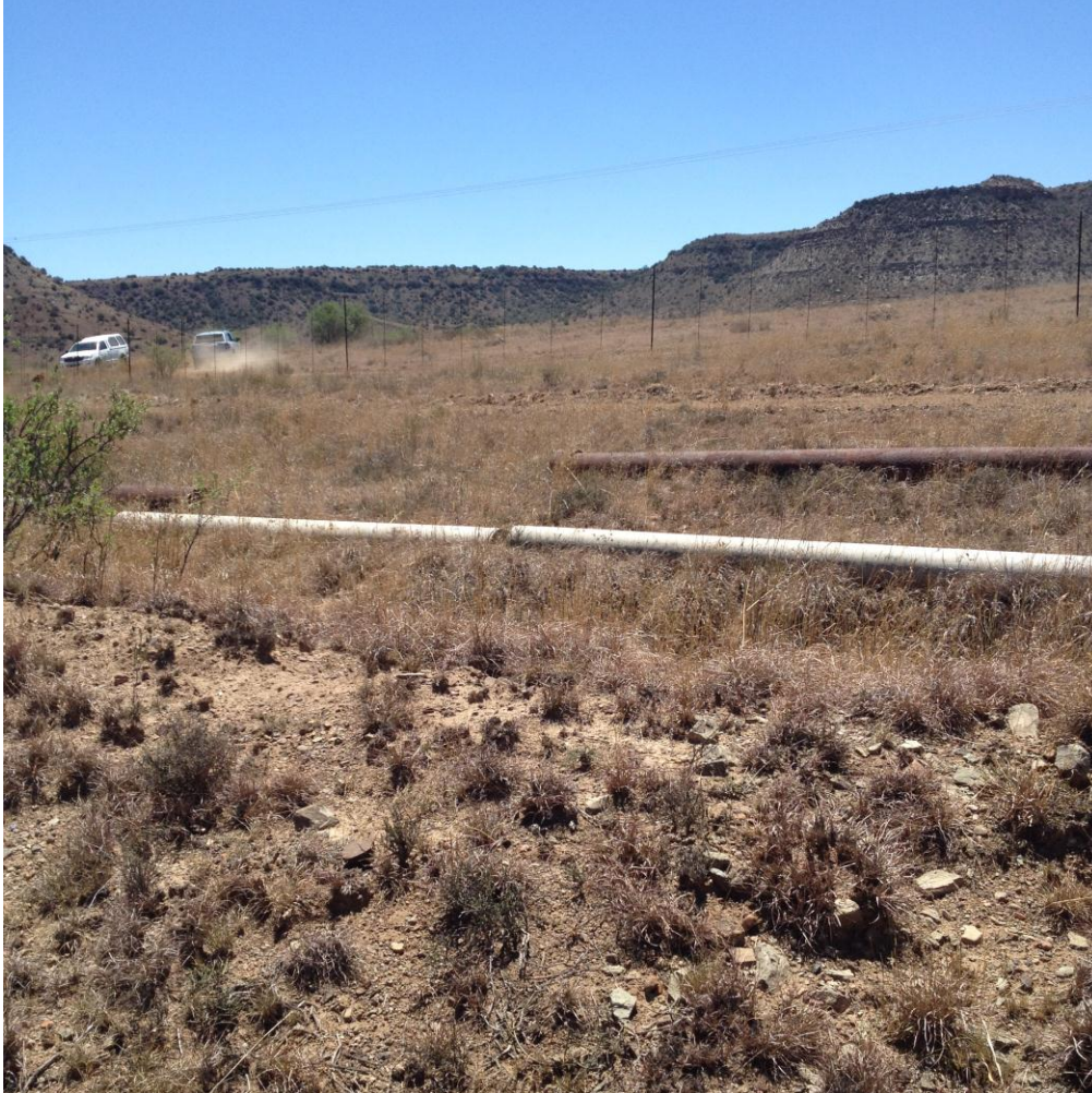
Image 12: Old pipe line infrastructure to feed water into the close by man-made dam
