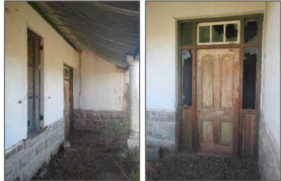
Figure 7-74: Porch and front door details at the front of the main house at waypoint 1791 in HL04.
