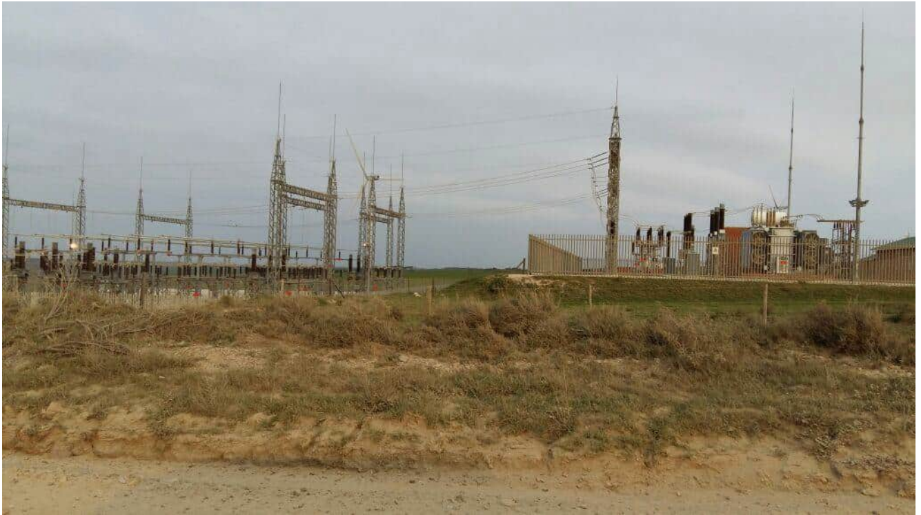
Figure 2-14: Example of a Wind Farm Substation (right) and adjoining Eskom Switching Station (left) on the Kouga Wind Farm
