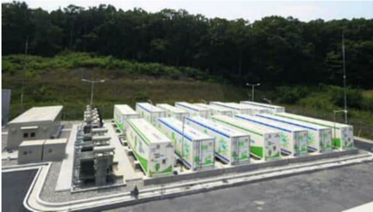
Figure 2-15: Example of a Lithium-Ion BESS installation
