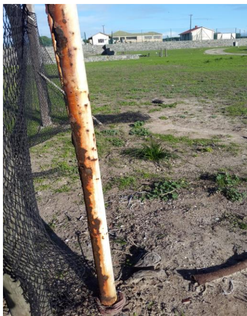
Figure 4: The current look of the rugby posts at the Village Precinct Stadium
