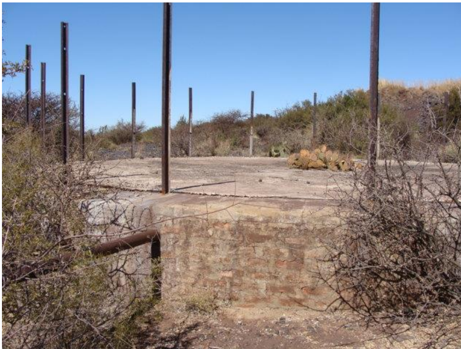
FIGURE 43: REMAINS OF A WATER RESERVOIR.
