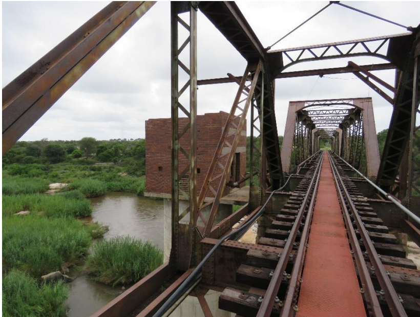
FIGURE 30: THE PUMP HOUSE ON THE BRIDGE. THE PUMP HOUSE DATES TO THE LATE 1950'S/ EARLY 1960'S AND THEREFORE IS YOUNGER THAN 60 YEARS OF AGE. HOWEVER, IT DOES NOT HAVE ANY HERITAGE SIGNIFICANCE.
