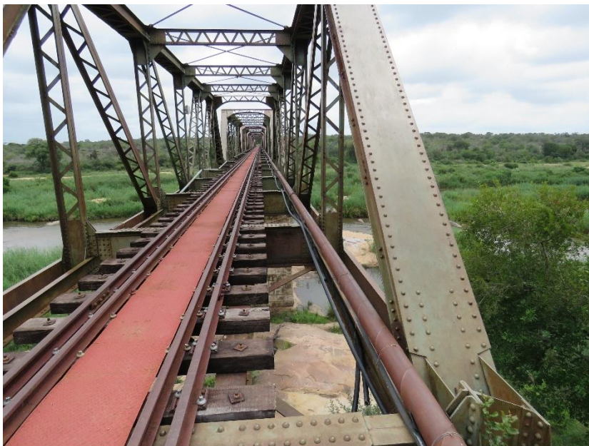
FIGURE 29: NOTE THE PIPE ON THE RIGHT-HAND SIDE AS WELL AS CABLES, AN INDICATION OF LATER, BUT REVERSIBLE ADDITIONS TO THE BRIDGE.
