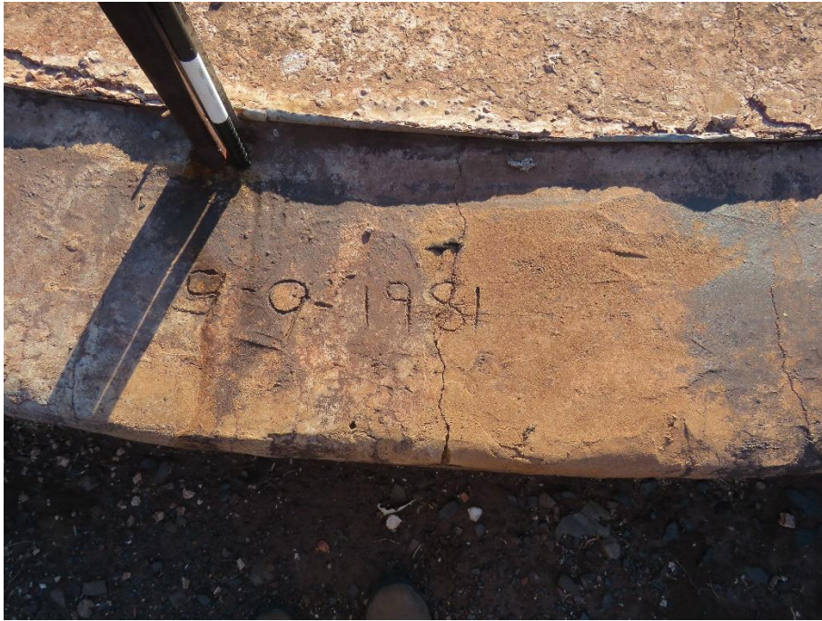
FIGURE 53: DATE INSCRIBED IN THE CONCRETE.
