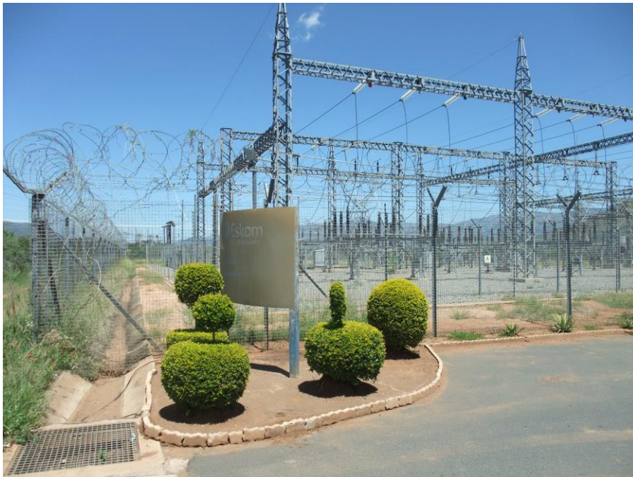
Figure 5: The Merensky substation.
