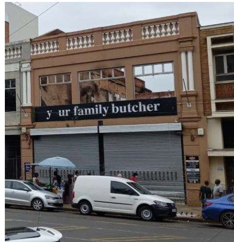
Figure 2: 287 Church Street After Fire Damage
