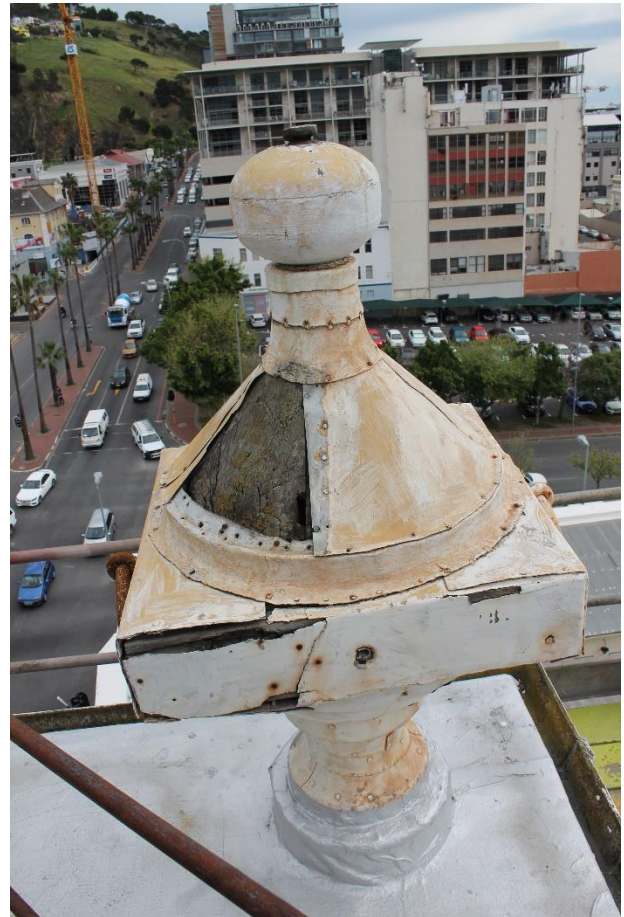
The third urn showing loss of metal cladding and serious rot in the top and centre section with the additional loss of one of the cast iron rings from the side.
