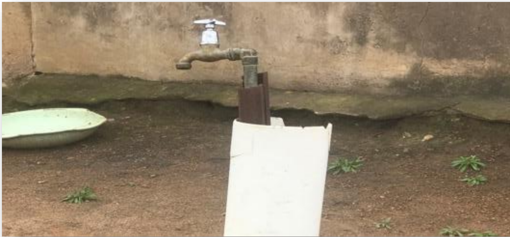
Figure 26: Piped water in compound
