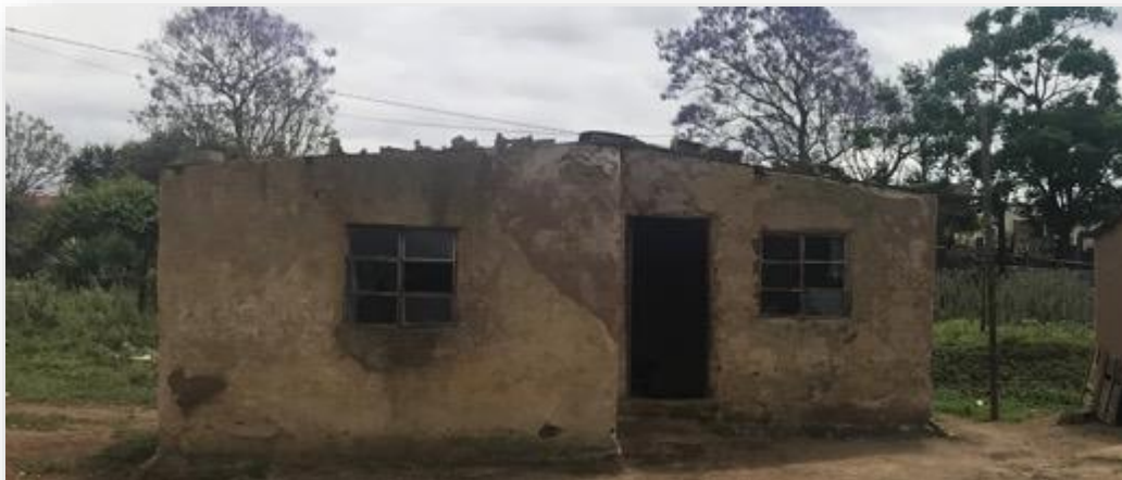
Figure 15: Example of house in poor condition
