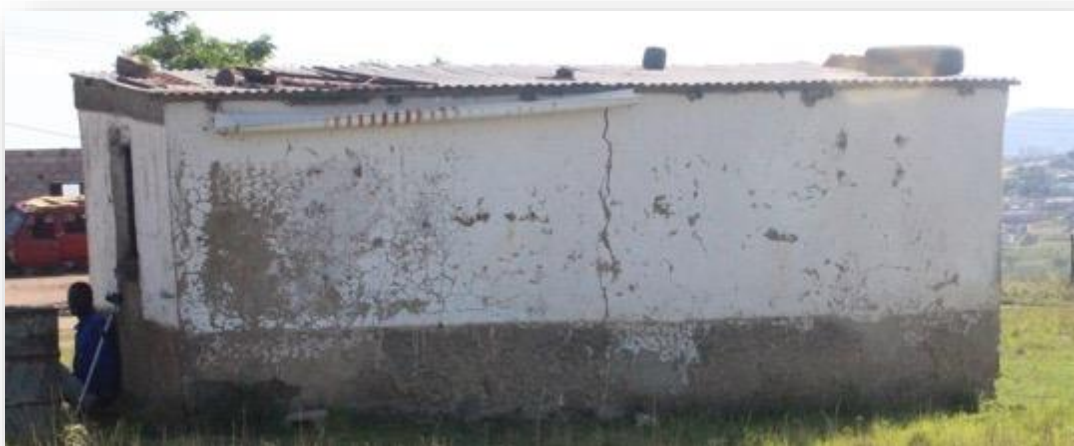
Figure 17: Example of house in poor condition
