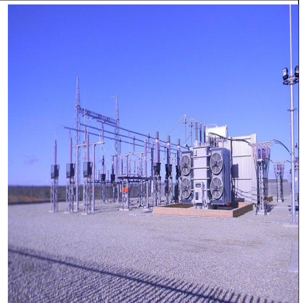
Figure 7.4: Substation (Eskom Sere Wind Facility)
