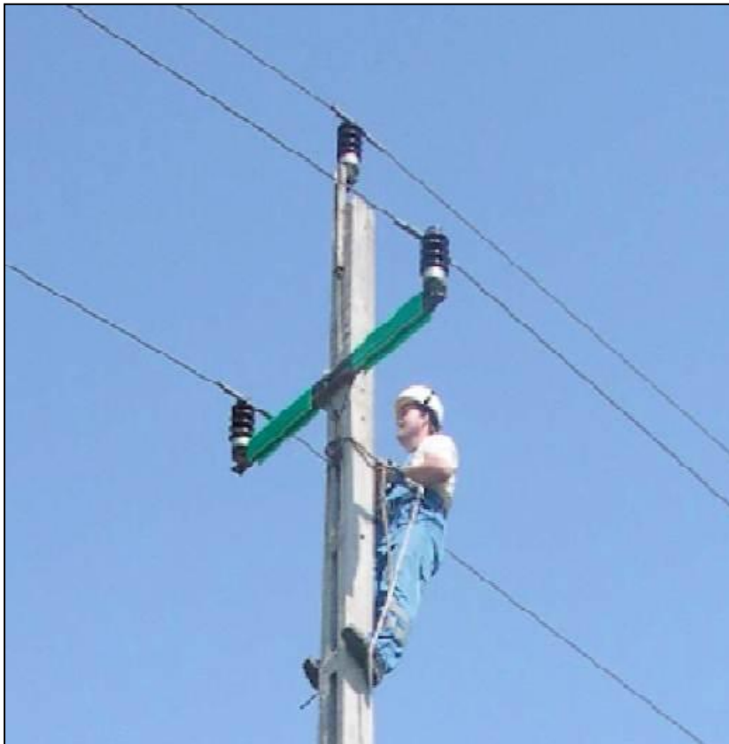
Photograph 3. Cross-arm insulation (source: Horvath et al., 2011)
