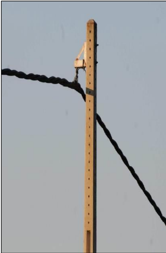
Photograph 5. Completely insulated medium tension cable hanging from concrete pole without need of insulators (source: Haas, 2011)
