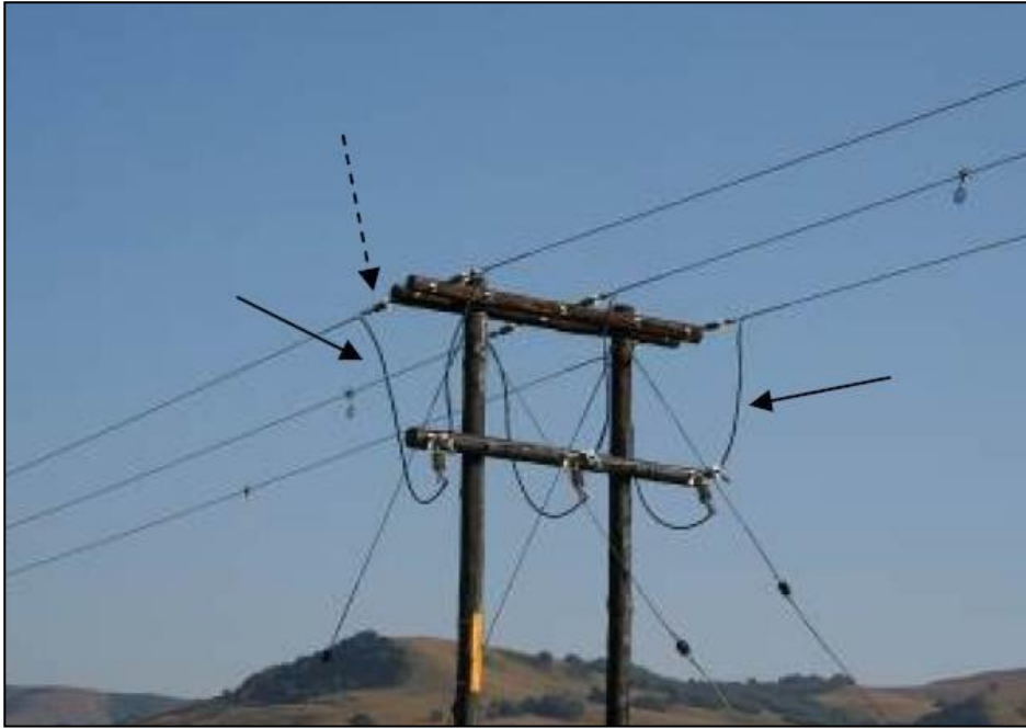
Photograph 4. A safe strain pole structure, with insulated jumper wires (black arrows) and sufficiently long insulators (broken arrow) (Photo: EWT-WEP)
