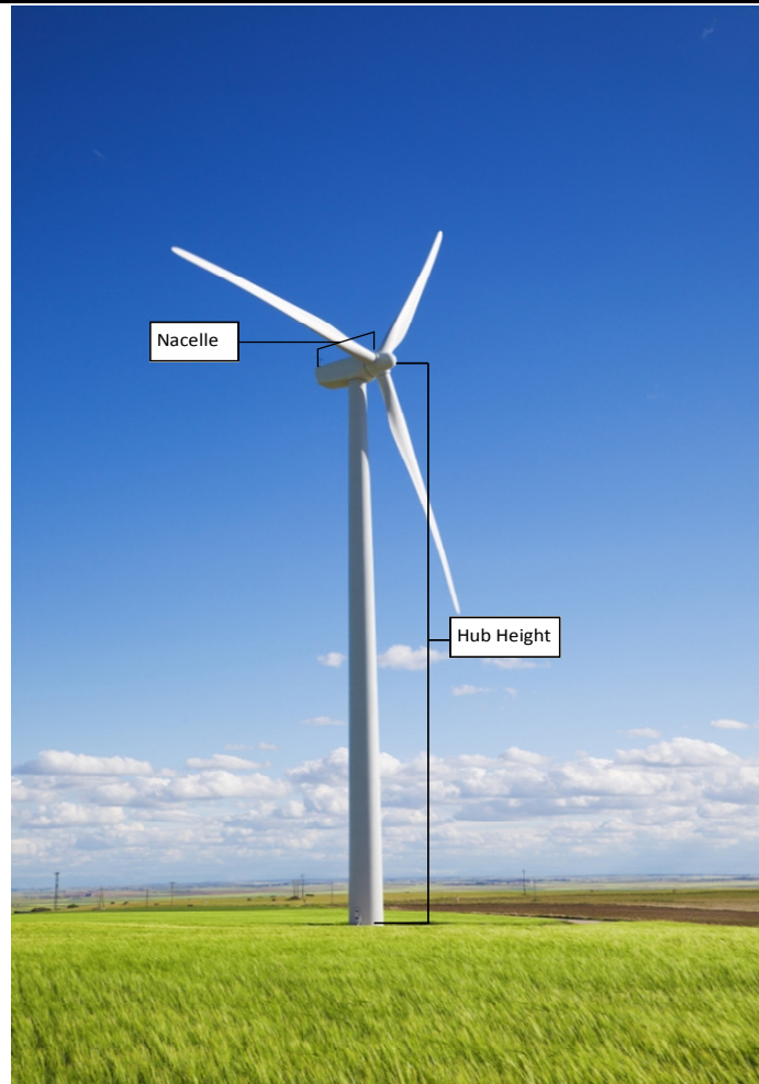
Figure 0.2 Typical Wind Turbine
