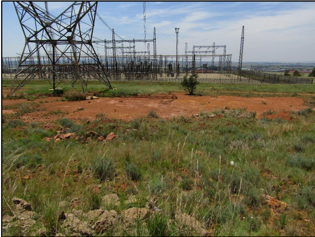
Figure 21: Footprint of the existing pylon at Etna substation. Vegetation cover must be reinstated following installation of pylons.
