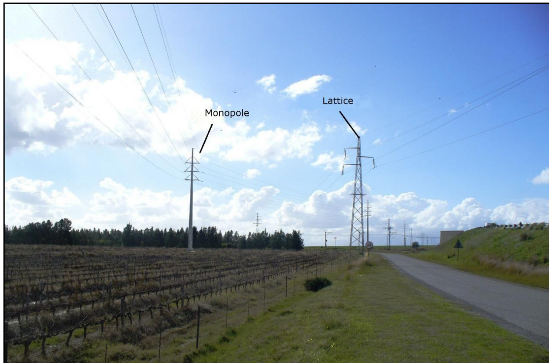
Figure 3: Typical 132 kV power line structures
