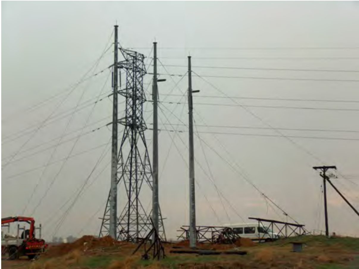
Figure 1-23 An example of monopole towers next to a lattice type tower for 132 kV power lines. (Source: http://www.rame.co.za/flagship-projects/132kv-lattice-to-mono-pole-replacement/nggallery/image/578 )
