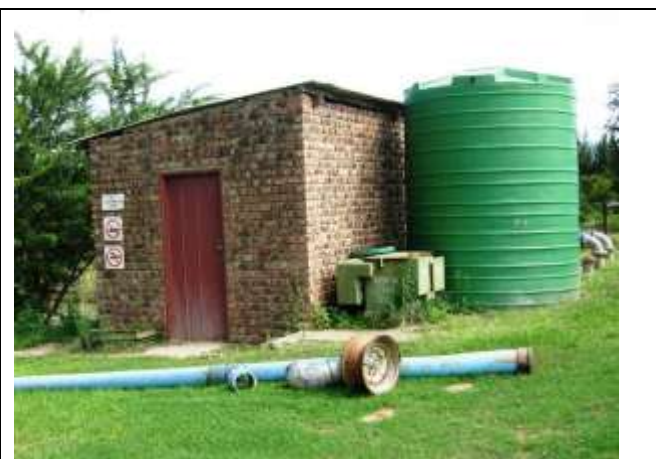
Photo 2.6. Pumping infrastructure at an existing dam (pump-house & transformer).
