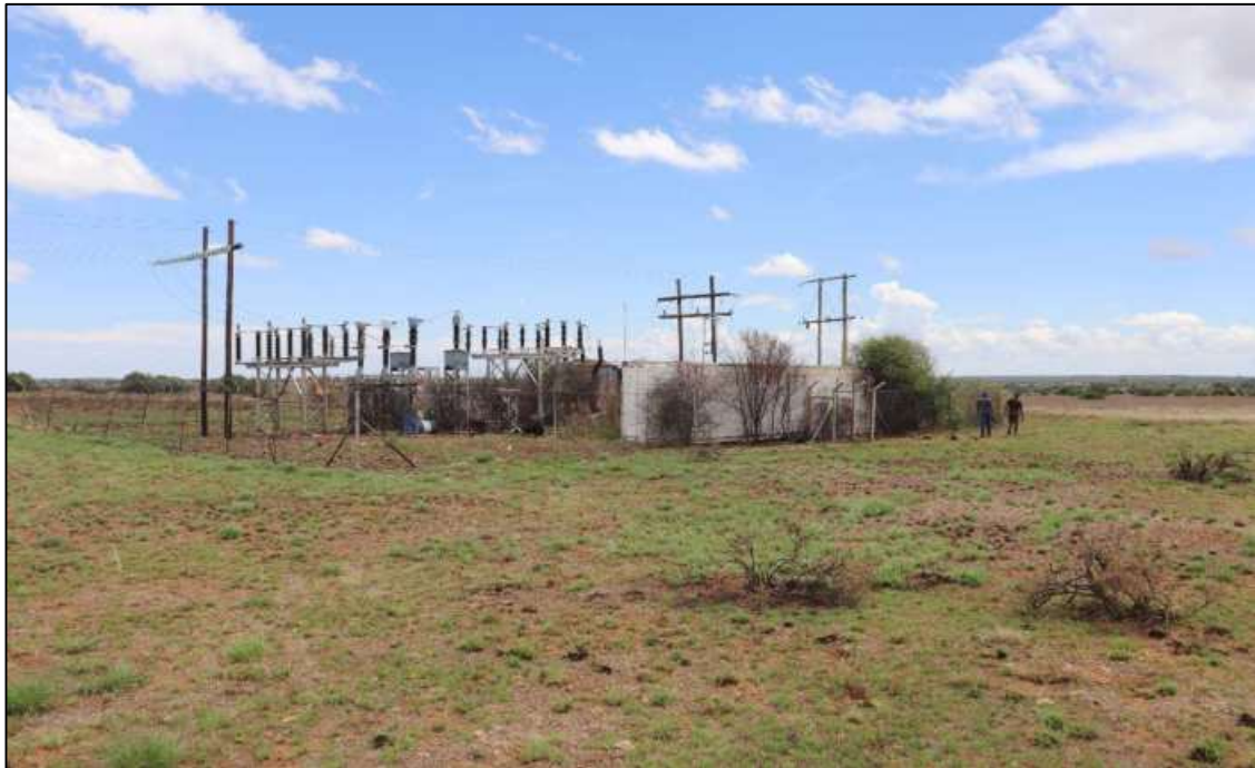
Figure 4: Existing power substation on the property
