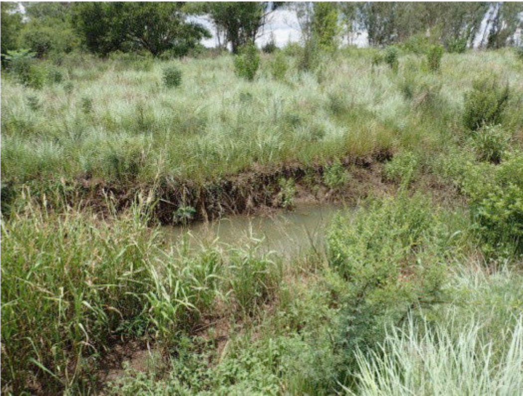
Figure 26 Eroded channel along the watercourse
