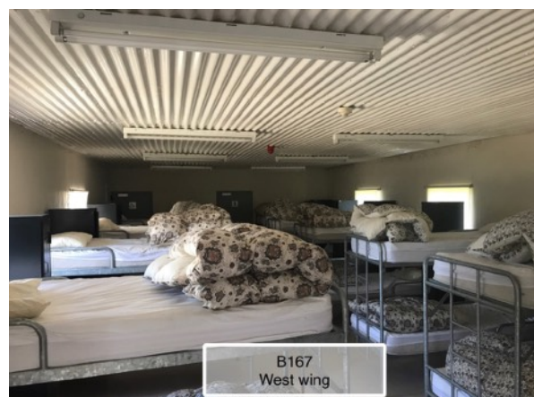
Fig 6. Note the flaking paint on the walls close to the concrete ceiling. Most likely caused by excessive moisture generated by children with walls not being able to 'breathe'.
