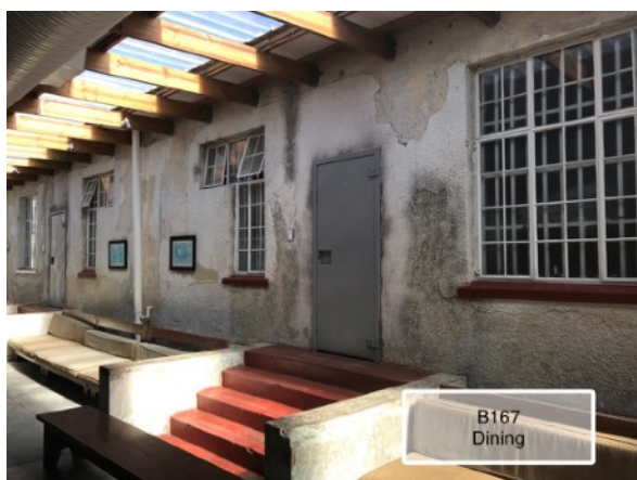
Fig 5. Black mould on walls in dining area. Causes need to be established
