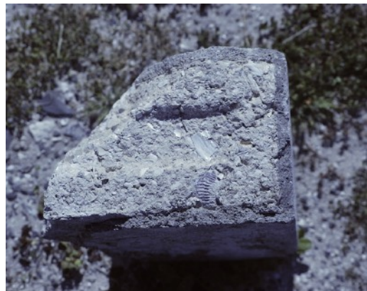
A sample of limestone brick found on Robben Island. A typical example of the quality of brick produced. It appears if the mortar contains cement, which should be analysed to determine the mortar mix for the restoration work.
