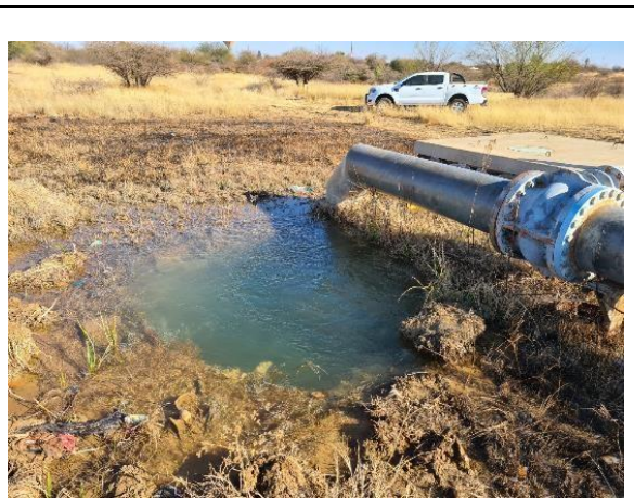
Photograph 10-4: Leaking pipeline in the north-eastern section of the Roodepan site
