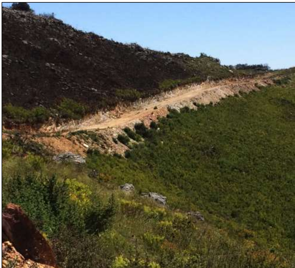
Figure 6-2: A cut and fill road, with a footprint extending further than the 6m road width.
