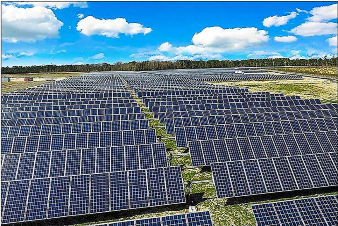
Figure 2.1: Typical example of solar PV array
