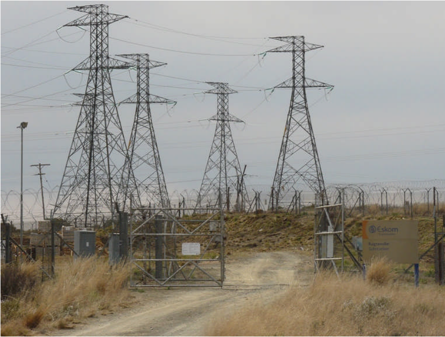
Plate 1 Ruigtevallei substation near the Oviston Dam wall.
