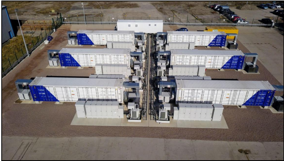
Figure 3: Aerial view of a BESS (Photo: Power Engineering International)
