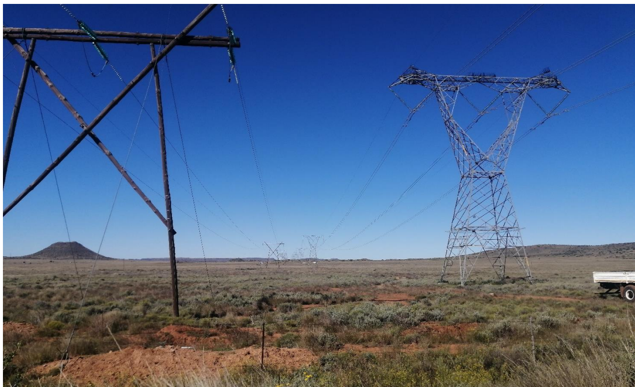
Figure 10: Electrical infrastructure that traverses the study area
