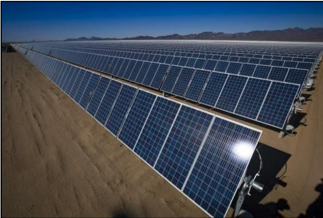
Photograph 1.1: Typical PV SEF facility
