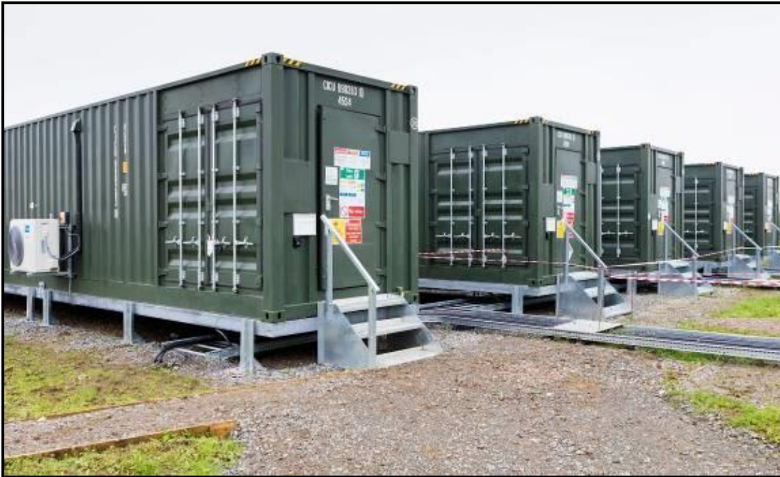
Photograph 1.2: Example of BESS located in storage containers
