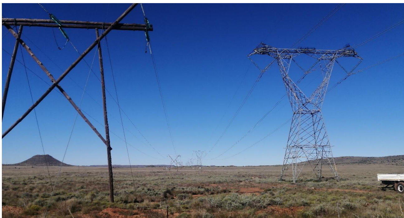
Figure 11: Electrical infrastructure that traverses the study area
