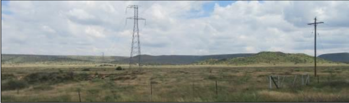
Photograph 3.4: Transmission line on Ruspoort
