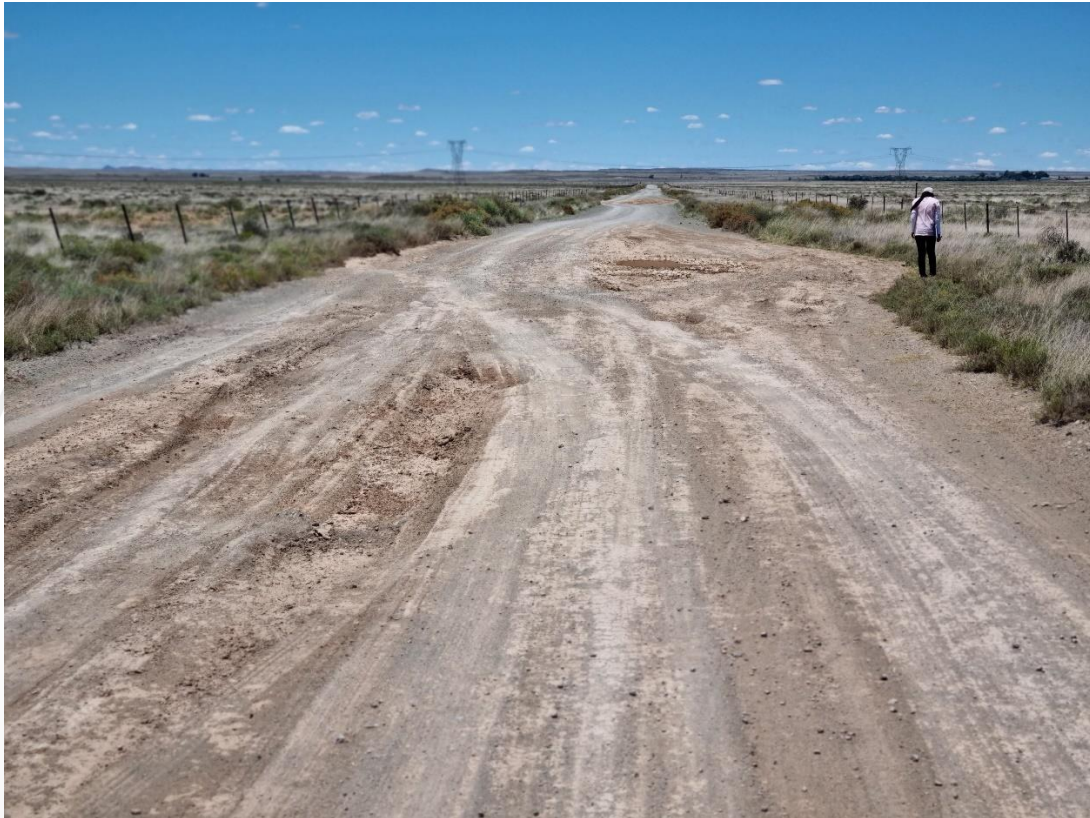
Photo 19. A Geotechnical Assessment will be undertaken to determine the founding stability and extent of reconstruction required on the public (above) and private sections of road.
