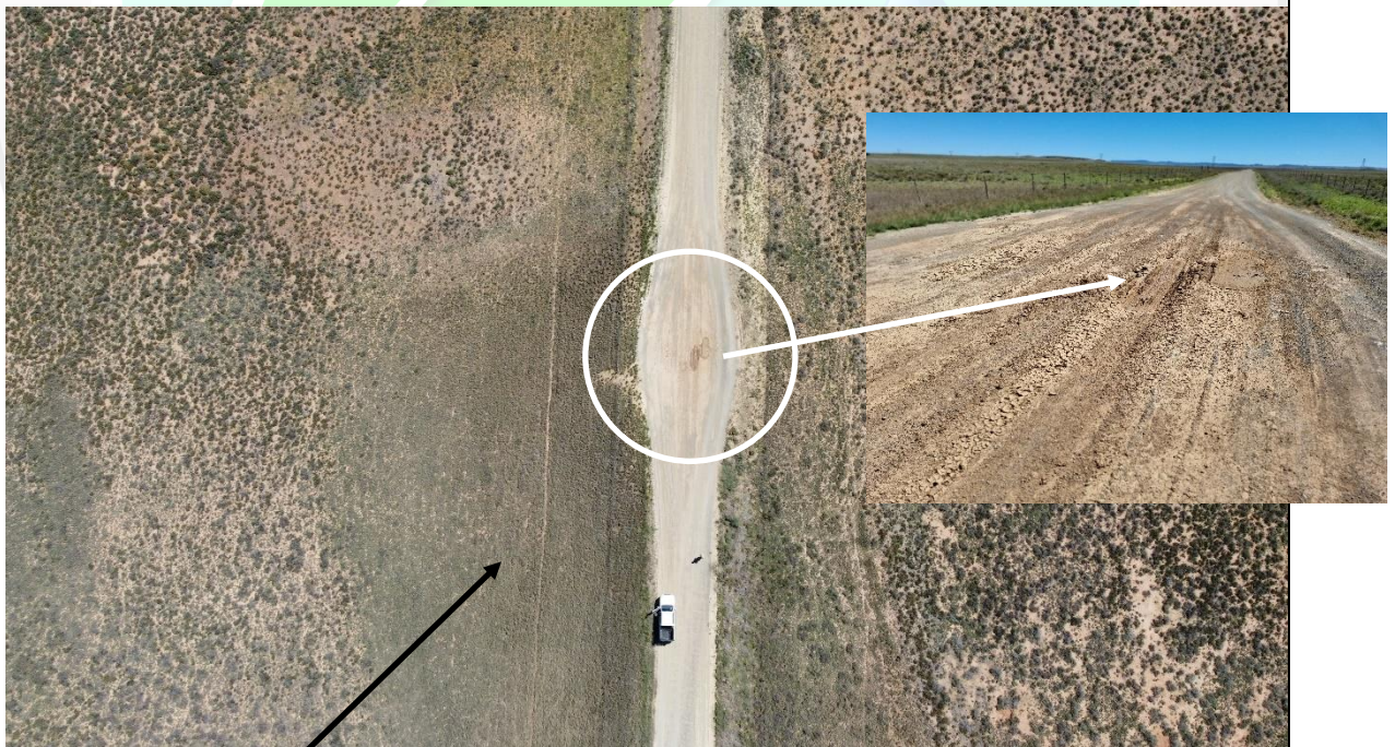
Photo 10. Possible seep (and associated road failure) adjacent to the servitude of the public 'Burgerville' District Road (2448).
