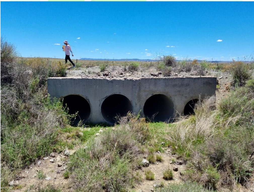
Photo 11. There is an existing pipe culvert (9 m wide shoulder width) on the public district road section.
