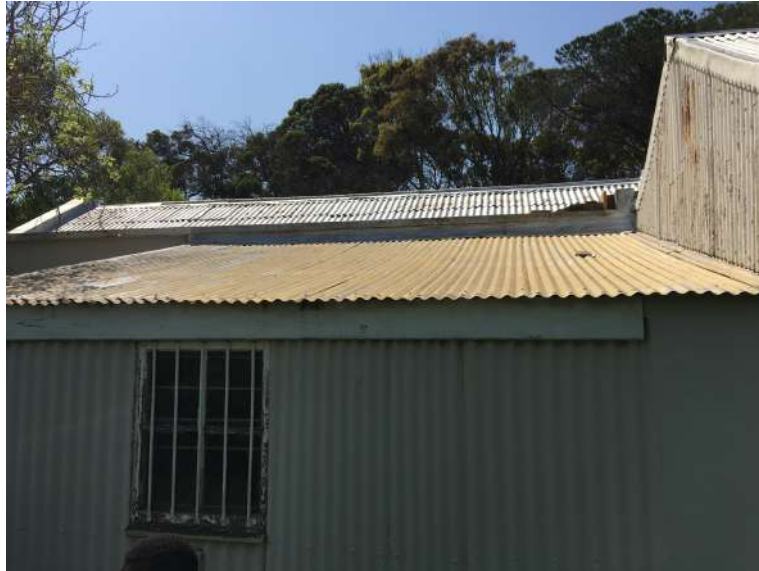
Fig. 3 - Sagging of roof on corrugate clad addition on north-western corner.
