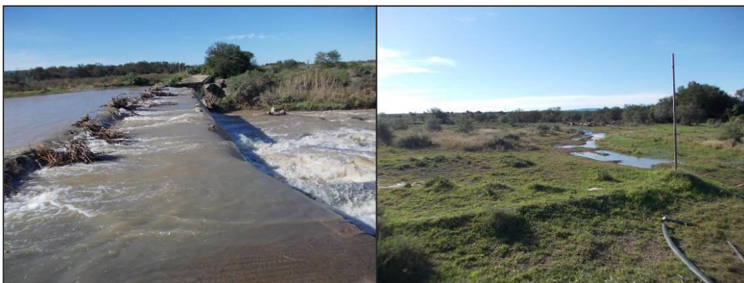
Figure 18: Degraded, flooded bridge structure associated with site 12 (left) and seepage from dam (right).
