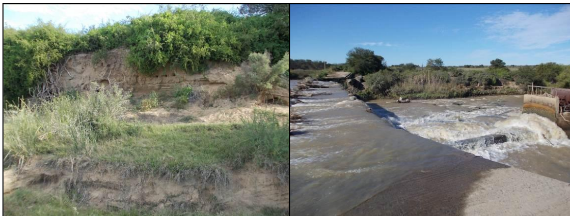
Figure 20: Erosion and incision of river banks (left) and bridge structure within the active channel of the river (right).
