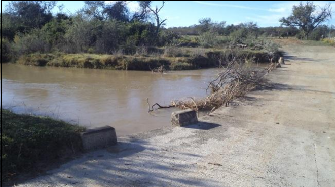
Figure 26: Upstream view of Site SM1 showing bridge infrastructure. The bridge is currently operational.
