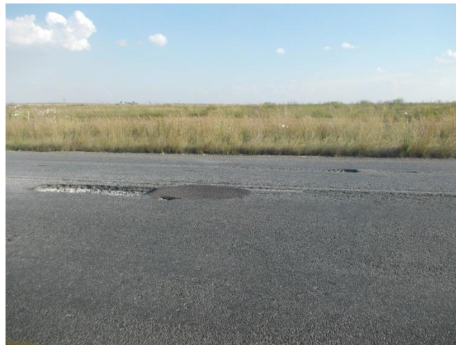
Figure 22: One of many deteriorated sections along the R29 roadway
